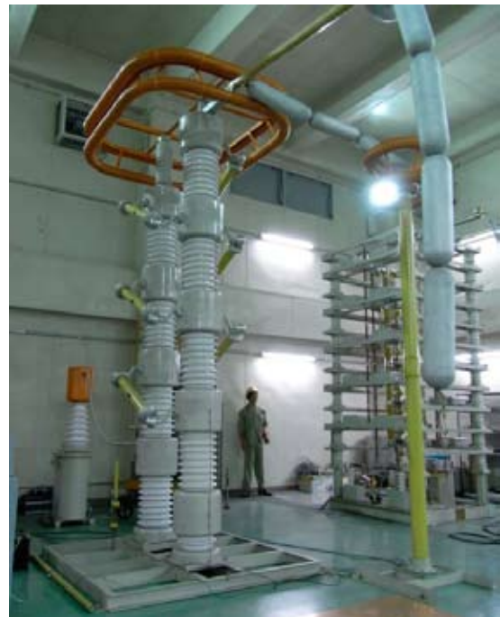
High-voltage facility for the prevention of electric shock hazards.
