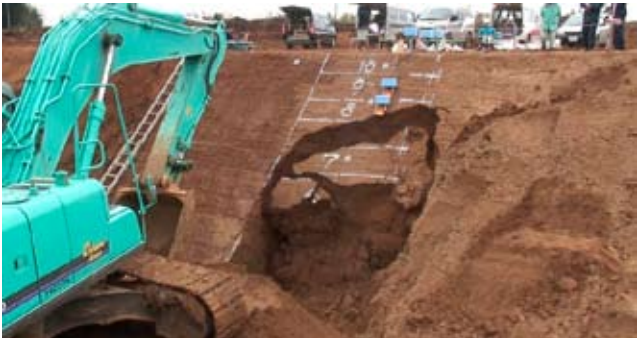
Experimental study for investigation of the mechanism of slope failures.
