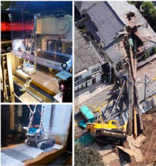
Study on potential risks of overturning of drill rigs being self-propelled over unstable ground at construction sites.
