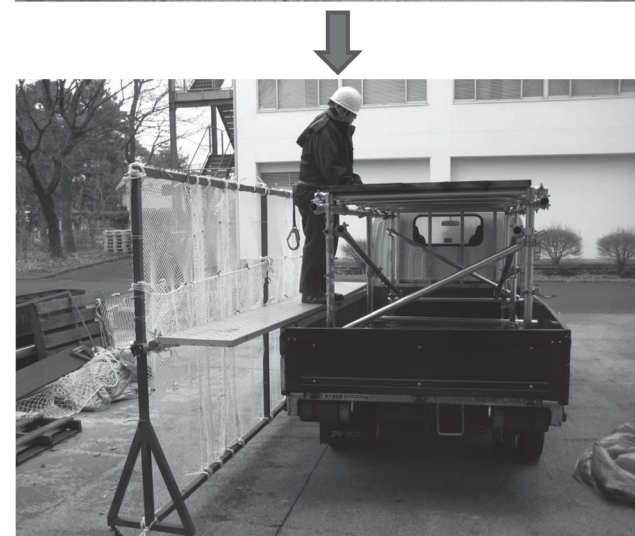
Fig. 13. Work stage developed by the JNIOOSH for preventing falls during cargo-handling operations.
