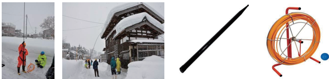
Figure 2. (Left) Rakubo at work in rooftop snow removal. (Right) Rakubo stick, pilot line.
